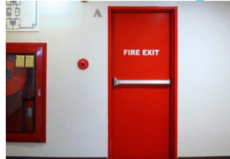
STEEL DOORS FIRE AND NON-FIRE RATED.
